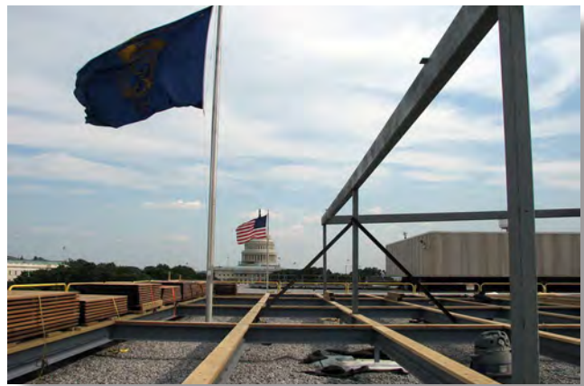
In late June, the construction workers get busy laying the support for the wood decking.
