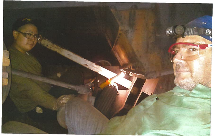
Hard at work aboard the SS MATSONIA are 2nd A/E Matt Ramos and Jr. Engineer Greg Cavan plugging tubes in the steam drum.
